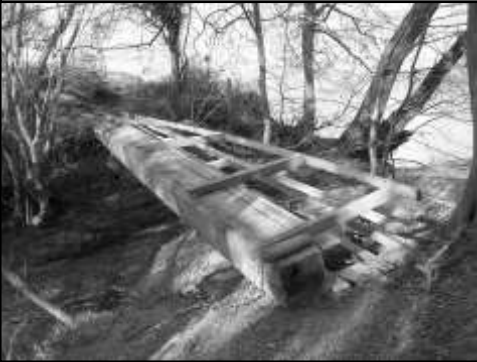
The collapsed Shellbrook Bridge
